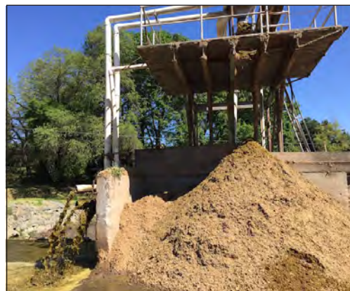
Screw auger separation of liquid and solids
