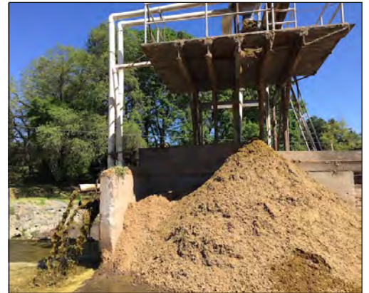
Screw auger separation of liquid and solids
