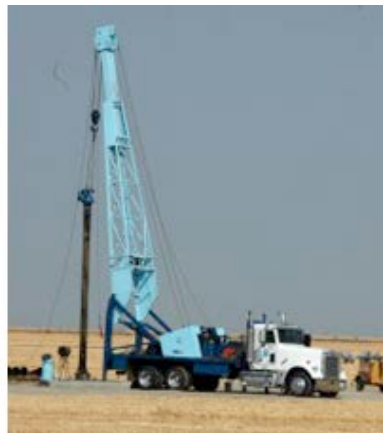
Faced with no surface water supplies, many growers have had wells drilled.
