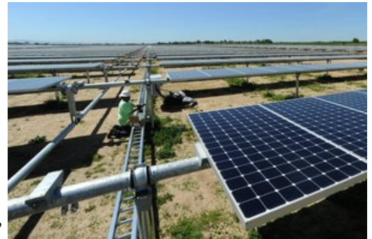
(Debbie Noda/dnoda@modbee.com) The Solar project is being installed at McHenry Ave. and Patterson Rd., April 19, 2012. - Modesto Bee - Debbie Noda
